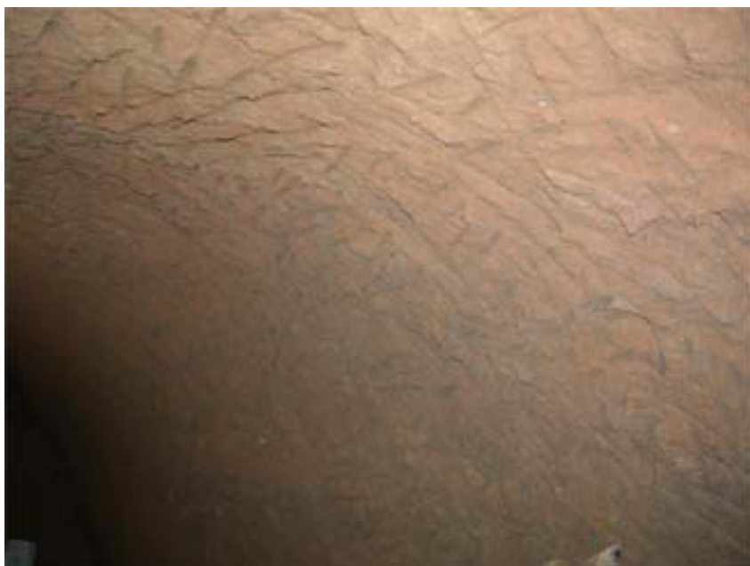
FOTO 97: Entrada 5/Tram9, marques instruments
